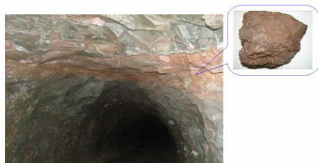
图 1 层间错动带在白鹤滩水电站水平探洞中的出露示例 Fig.1 An example of interlayer shear weakness zone from an exploratory tunnel of Baihetan hydropower station
