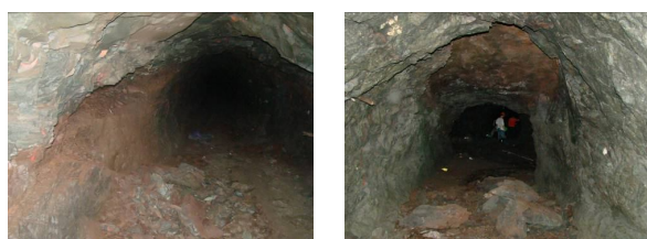
(a) 边墙开裂
